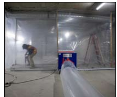
Worker drilling concrete inside an enclosure equipped with a “negative air” unit
